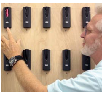
HAI's Ernie Sieber, Technical Support Supervisor, inspects HAI Access Control Readers.
