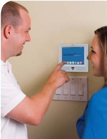
Touchscreens throughout the home provide easy control of a variety of home systems.
